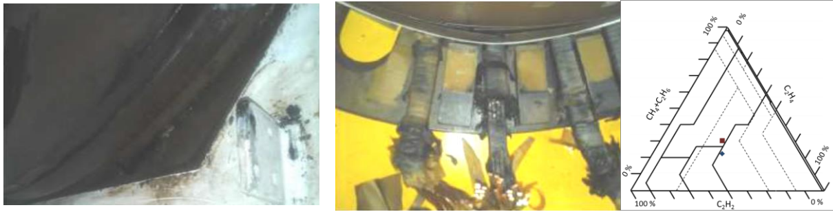
Figure 9 – Flashover marks, overheating and triangle
