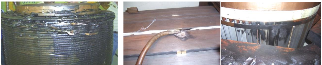
Figure 12 – Electrical discharges and overheating
